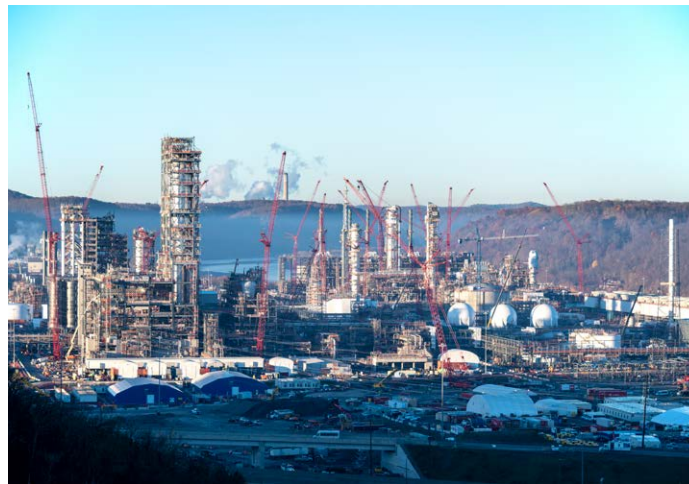
Construction of the Shell Pennsylvania Petrochemicals Complex in the US (2020). Robert Michaud, iStock.
