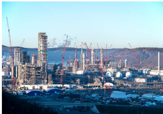
Bau des Shell Pennsylvania Petrochemicals Complex in den USA (2020). Robert Michaud, iStock.
